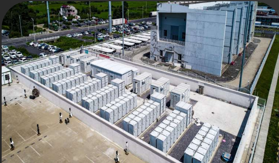
Energy Storage Project on User Side of Jiangsu Contemporary Amperex Technology Limited
